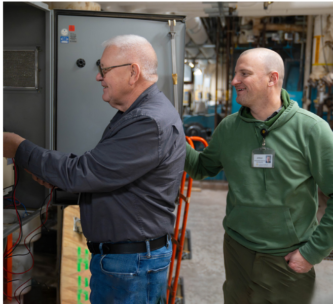
Maintenance engineers Jerrad Swanson and Mitchell Ehmke test the hospital's electrical panel.
