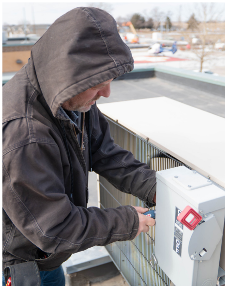
Maintenance engineer Travis Long examines rooftop machinery to confirm all equipment is operating efficiently.
